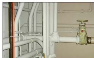
Piping and plumbing systems Photo by John M. Cimbala.
